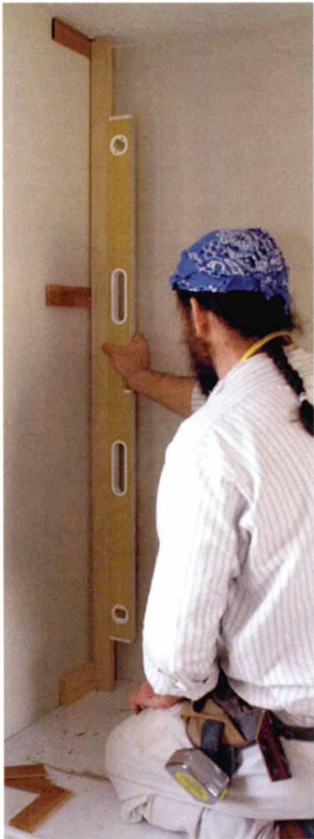
Shims set before the sides go in. Using a straightedge and a level, the author tacks shims to the wall to create a plumb line before the sides are fit.
