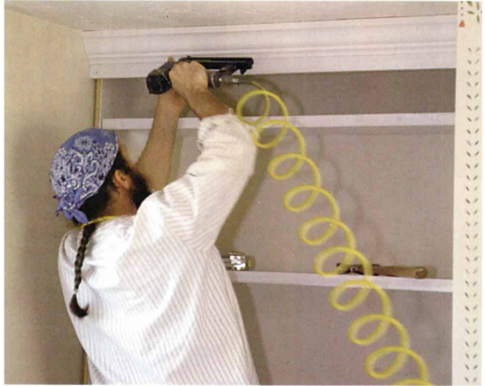
Crown hides ceiling discrepancies. The first trim to be installed is the crown backer and molding, which is adjusted to disguise a ceiling that is out of level.
