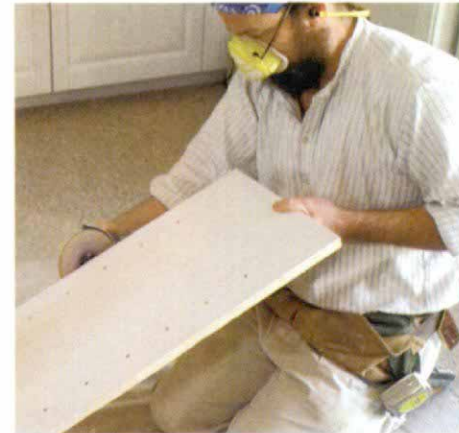
Grinding to the line. An electric grinder creates a bit of dust, but the grinder is easy to control and allows a feather edge to the scribe line.
